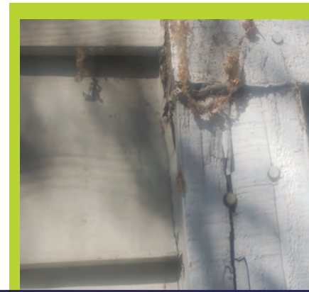
In this image, you can see the dry rotted wood trim adjacent to the cement fiber board siding.
